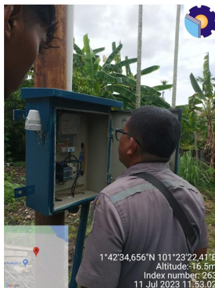
Gambar 2. 17 Pengecekan panel box
