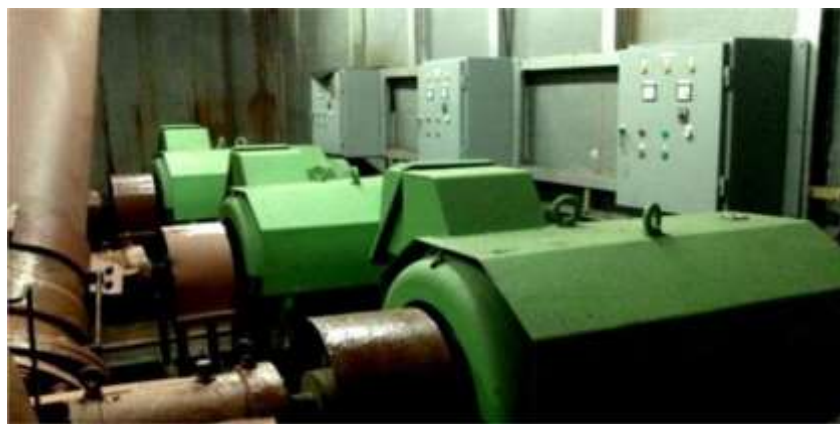
Gambar 1.7 Pompa Graving Dock
