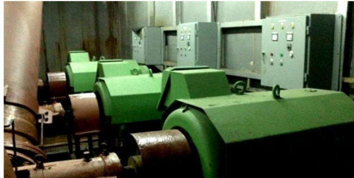
Gambar 1.6 Pompa Graving Dock
