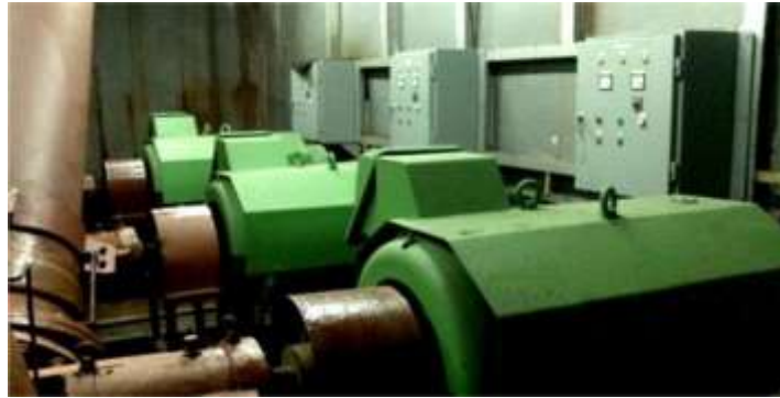
Gambar 1.6 Pompa Graving Dock
