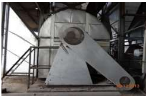
Gambar 3.134. Induced draft fan
