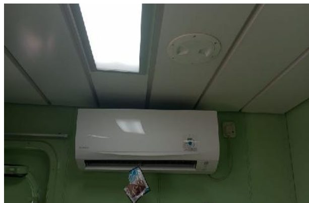
Gambar 3.9 AC Split Wall
