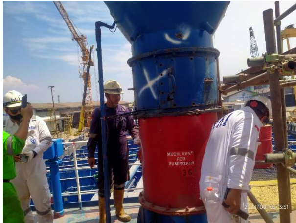
Gambar 2.24 Vent For Pumproom
