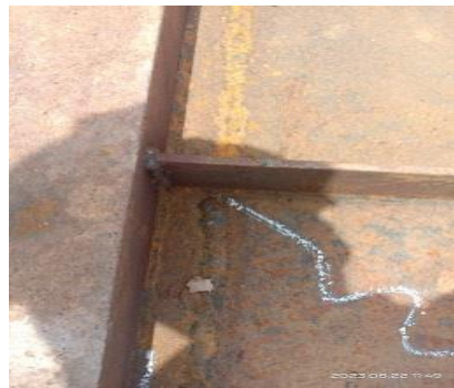
Gambar 1. 44 cacat welding undercut
