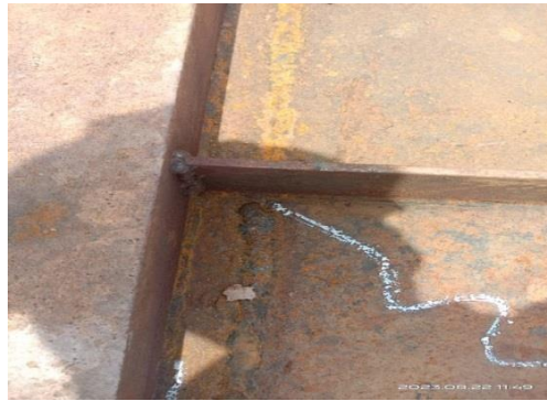
Gambar 1. 61 contoh cacat welding undercuts
