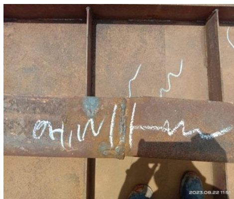
Gambar 1. 62 contoh cacat welding crack
