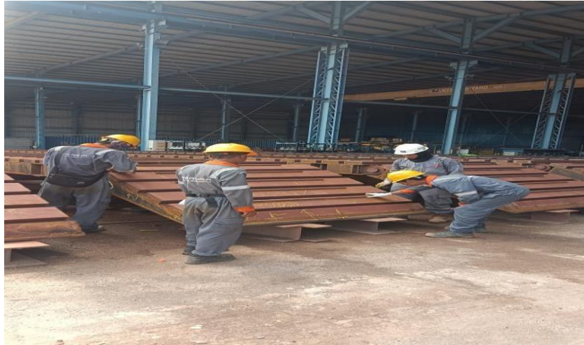
Gambar 2. 31 proses inspect ramdoor
