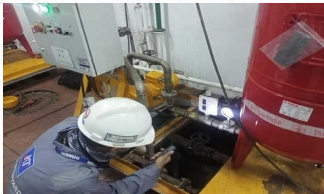
Gambar 2. 42 Pengecekan terhadap tekanan sistem fresh water pump
