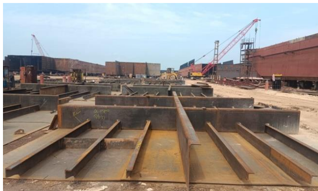
Gambar 2. 29 Panel main deck
