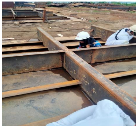
Gambar 2. 38 Pengecekan Cacat Las SAW
