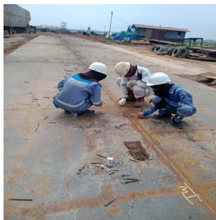
Gambar 2. 34 Pengecekan Cacat Las SAW
