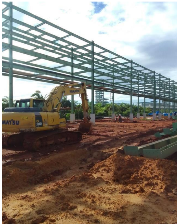
Comped tanah area compressor
