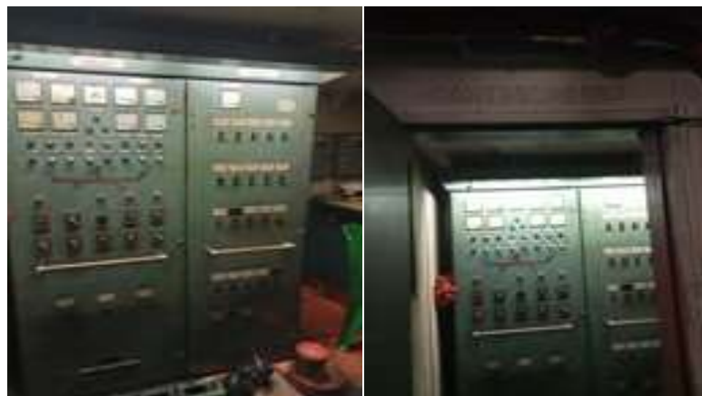
Gambar 2.52 Engine Control Room
