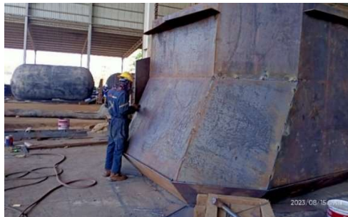
Gambar 2.36 Control Fitting Well House T.036 Louis Dolphin
