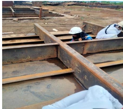
Gambar 2 54 Pengecekan cacat las SAW
