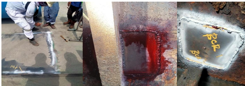
Gambar 2 36 developer, red penetrant, hasil kebocorannya
