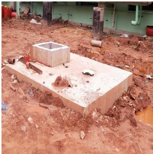
Gambar 2.17 Emergency Oil Tank
