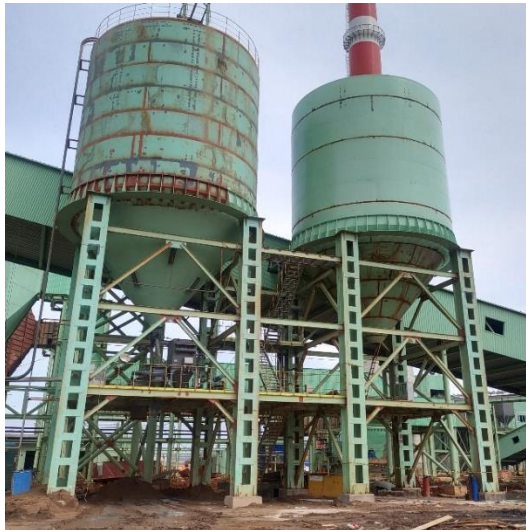
Gambar 2.19 .Fly Ash Silo
