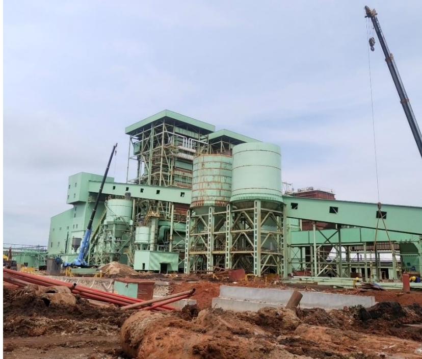
Gambar 2.2 Power Plant Sari Dumai Oleo (SDS2)
