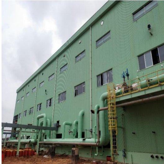
Gambar 2.24 .Main Power House
