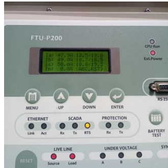
Gambar 2.18 Monitoring beban LBS ( Load Break Switch ) (Sumber: PT. Adra Gemilang)
