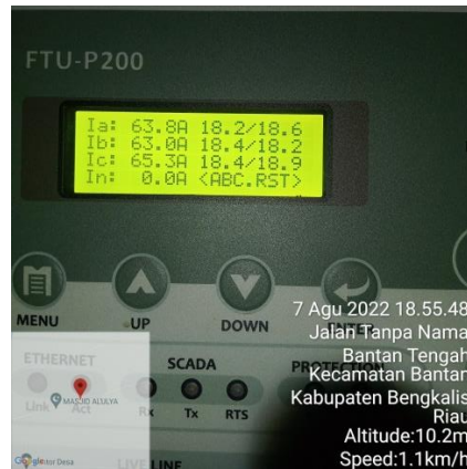
Gambar 2.40. Monitoring beban LBS ( Load Break Switch ) (Sumber: PT. Adra Gemilang)
