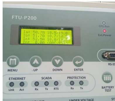
Gambar 2.25. Monitoring beban LBS ( Load Break Switch ) (Sumber: PT. Adra Gemilang)
