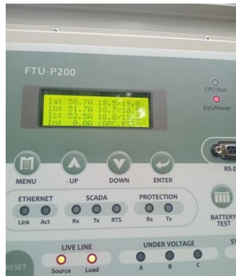
Gambar 2.3. Monitoring beban LBS ( Load Break Switch ) (Sumber: PT. Adra Gemilang)
