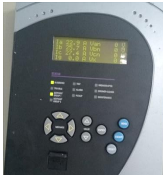
Gambar 2.55. Monitoring beban feeder (Sumber: PT. Adra Gemilang)
