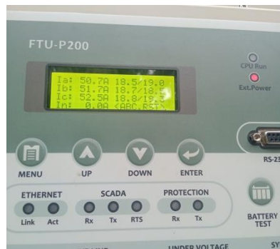
Gambar 2.30. Monitoring beban LBS ( Load Break Switch ) (Sumber: PT. Adra Gemilang)
