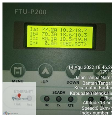
Gambar 2.54. Monitoring beban LBS ( Load Break Switch ) (Sumber: PT. Adra Gemilang)
