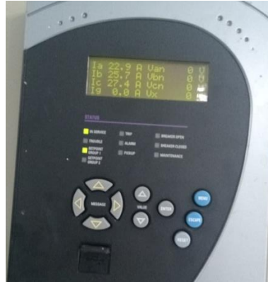
Gambar 2.28. Monitoring beban feeder (Sumber: PT. Adra Gemilang)
