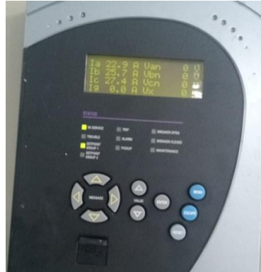
Gambar 2.43. Monitoring beban feeder (Sumber: PT. Adra Gemilang)
