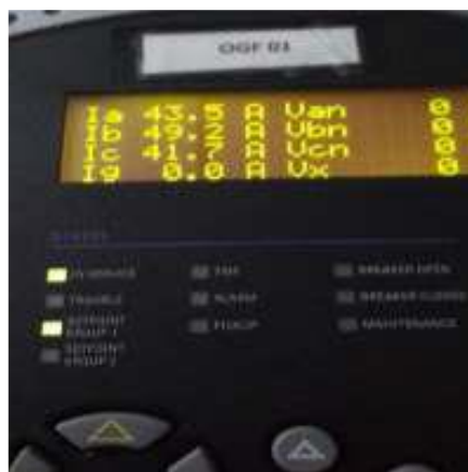
Gambar 2.12 Monitoring beban feeder (Sumber: PT. Adra Gemilang)
