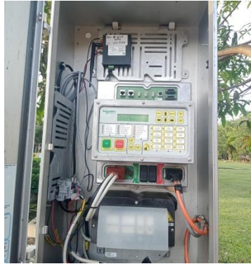
Gambar 2.21. Monitoring beban RC ( Recloser ) (Sumber: PT. Adra Gemilang)
