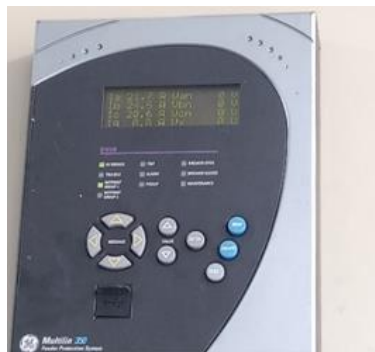
Gambar 2.9. Monitoring beban feeder (Sumber: PT. Adra Gemilang)
