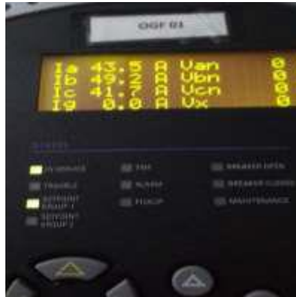
Gambar 2.24. Monitoring beban feeder (Sumber: PT. Adra Gemilang)
