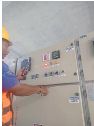
Gambar 2.14. Monitoring beban feeder (Sumber: PT. Adra Gemilang)
