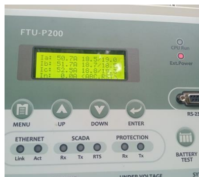
Gambar 2.22. Monitoring beban LBS ( Load Break Switch ) (Sumber: PT. Adra Gemilang)
