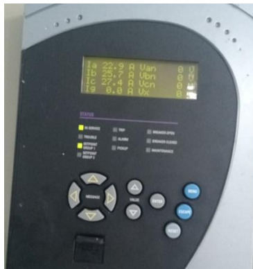
Gambar 2.48. Monitoring beban feeder (Sumber: PT. Adra Gemilang)
