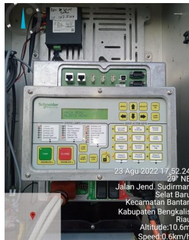
Gambar 2.52. Pengecekan baterai dn modem wifi Recloser (Sumber: PT. Adra Gemilang)
