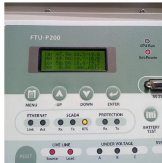
Gambar 2.7 Monitoring beban LBS ( Load Break Switch ) (Sumber: PT. Adra Gemilang)
