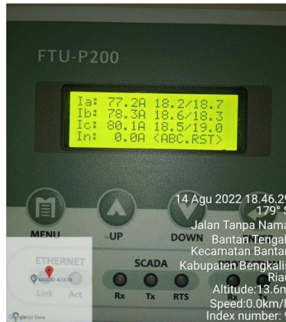
Gambar 2.49. Monitoring beban LBS ( Load Break Switch ) (Sumber: PT. Adra Gemilang)
