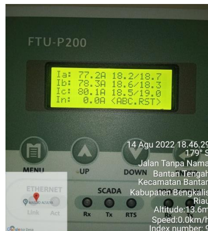
Gambar 2.45. Monitoring beban LBS ( Load Break Switch ) (Sumber: PT. Adra Gemilang)
