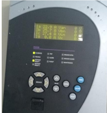
Gambar 2.31. Monitoring beban feeder (Sumber: PT. Adra Gemilang)
