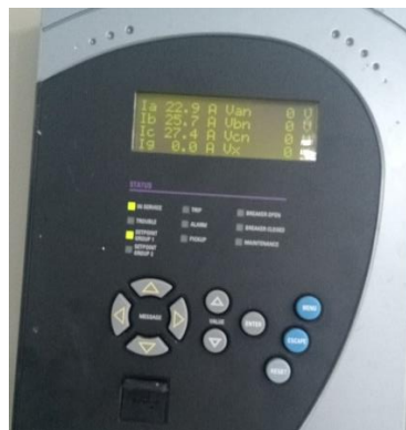
Gambar 2.36. Monitoring beban feeder (Sumber: PT. Adra Gemilang)
