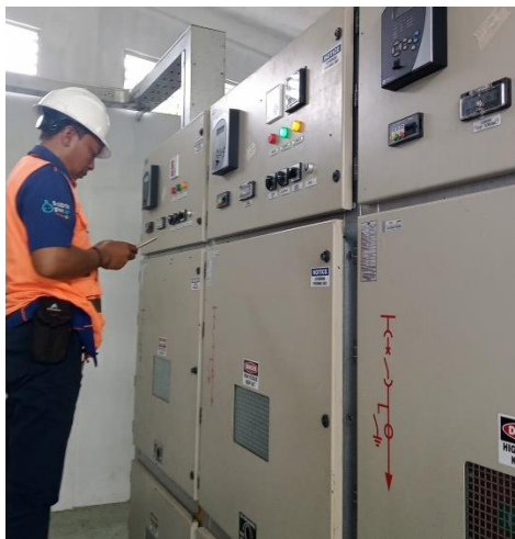
Gambar 2.33. Monitoring beban feeder (Sumber: PT. Adra Gemilang)
