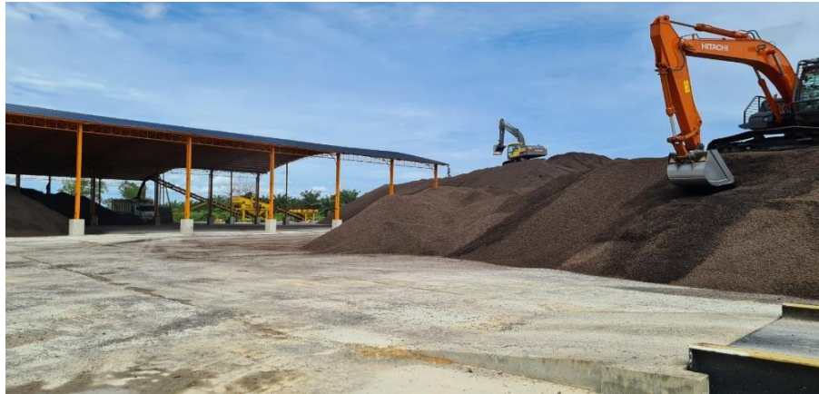
Figure 2.1 TanjungButon Stockpile Source: Tanjung Buton Stockpile
