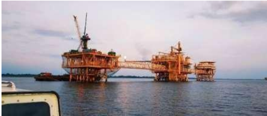
Figure 2.6 Lalang Well Platform
