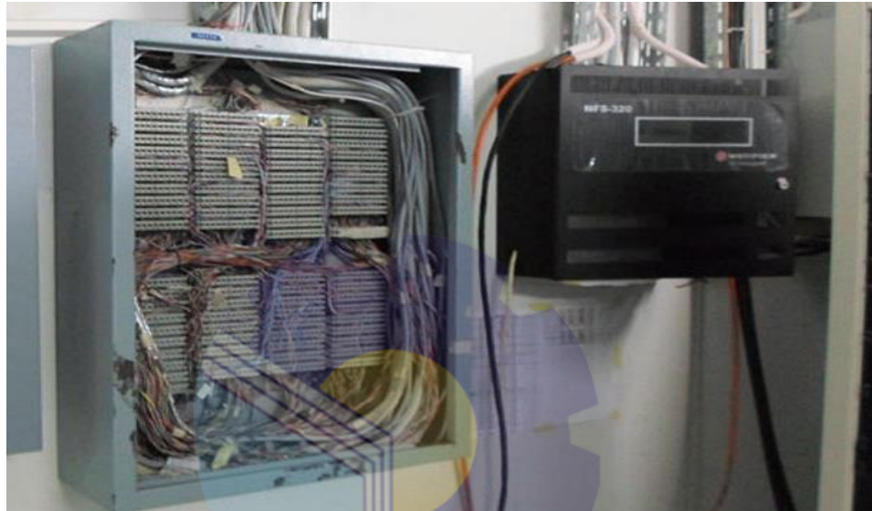
Gambar 1.1 Main Distribution Frame (MDF)
