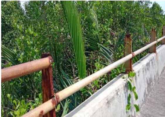
BESI RAILING HILANG
