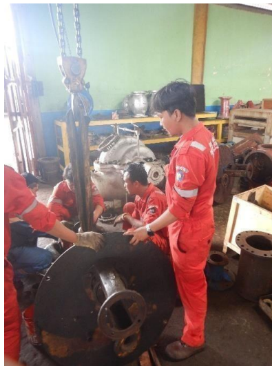
Gambar Lampiran2: Maintenance Vertikal Sump pump
