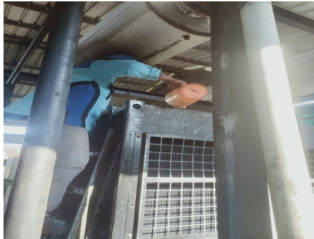
Gambar 2. 21 Kegiatan penambahan air radiator (Sumber: PT. Megapower Makmur Tbk. 2022)
