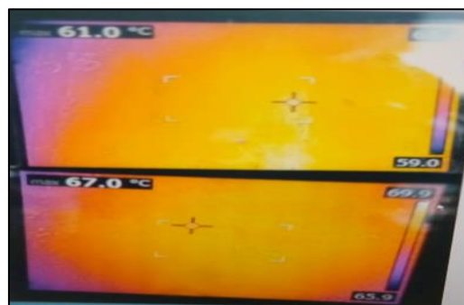
Gambar 4.20 Hasil Hotspot Termography
