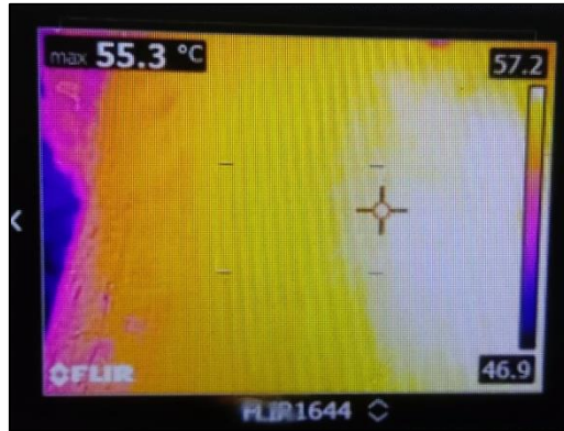
Gambar 4.21 Hasil Hotspot Termography
