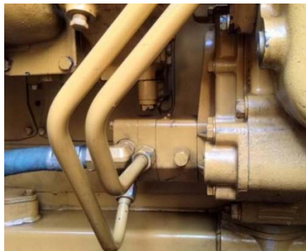
Gambar 4.4.4 Fuel Transfer Pump
