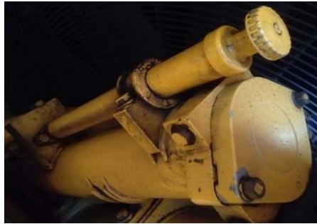
Gambar 4.4.5 Fuel Priming Pump Sumber: PT. PLN (Persero) PLTD II Bengkalis
