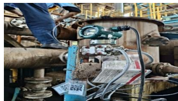
Gambar 2. 17 Ganti pres transmitter
