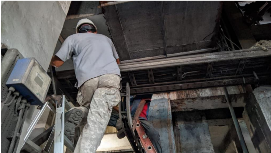
Gambar 2. 7 Perbaikan kabel ashenling Control Room Short plan LPB (Low Pressure boiler) (Sumber: Dokumentasi, 2024)
