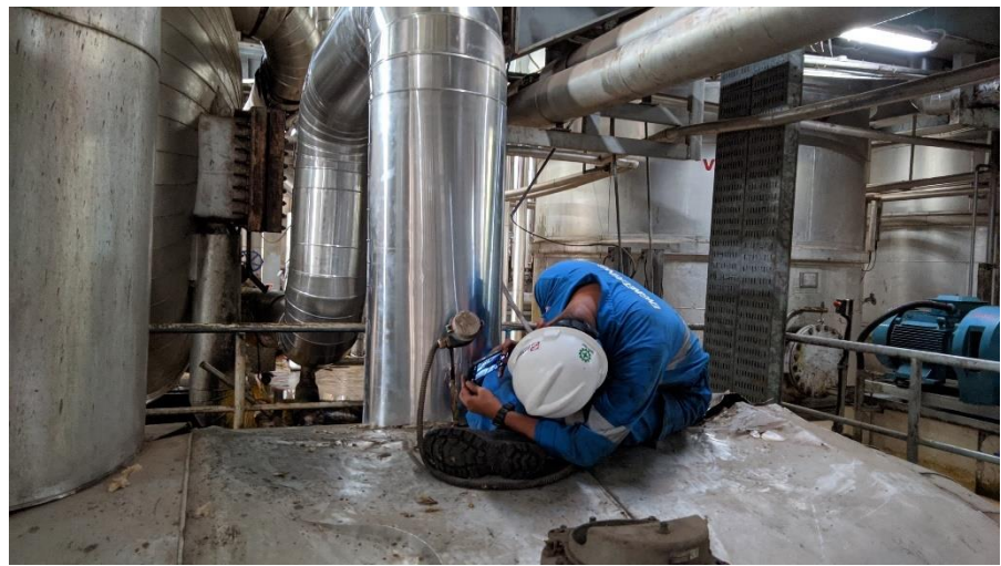
Gambar 2. 15 Pendataan serial number temperature transmitter endhauser di plan rifenery 1 (Sumber: Dokumentasi, 2024)
