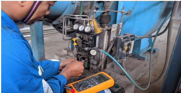
Gambar 2. 6 Perbaikan positioner ED FAN A di plan HPB ( High Pressure Boiler ) (Sumber: Dokumentasi, 2024)
