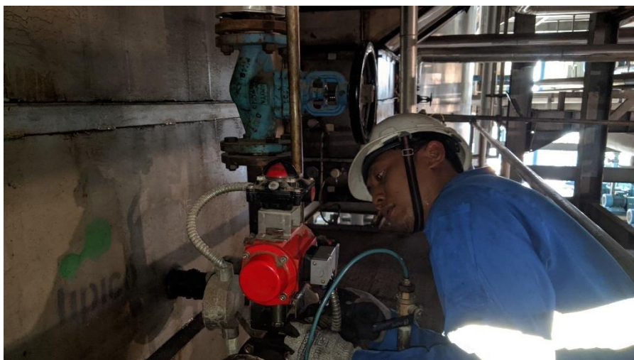
Gambar 2. 21 Pengecekan actuator valve line steam coil tank B filter press fraksinasi di refinery 1 (Sumber: Dokumentasi, 2024)
