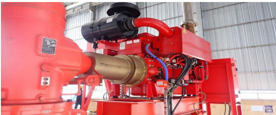
Gambar 4. 1 Fire Pump 717-PE-3
