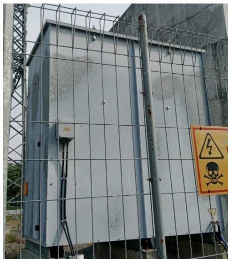
Gambar 3.7 Neutral Grounding Resitance (Sumber : Dokumentasi, 2024)
