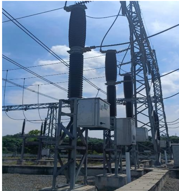
Gambar 3.5 CB ( Circuit Breaker ) (Sumber : Dokumentasi, 2024)
