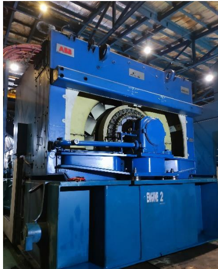
Gambar 3. 5 Generator sinkron PLTMG Duri
