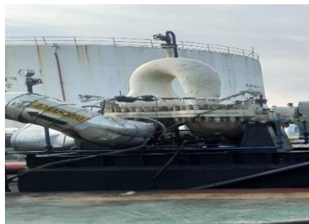
Gambar 4.2 pompa transfer feed pump 946-pm-1a
