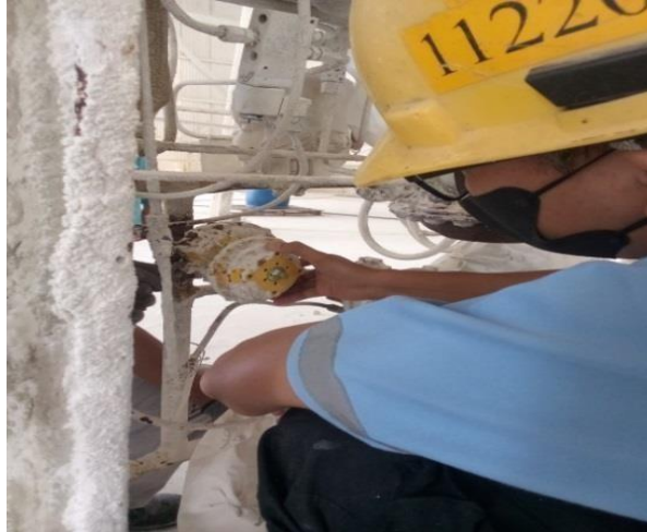
Gambar 2. 8 Servis Control Valve MFO(Marine Fuel Oil) burner (sumber ; Dokumentasi di PT. Indah Kiat Pulp and Paper)
