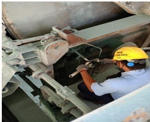
Gambar 2. 12 Servis tubing Bocor (sumber : Dokumentasi di PT. Indah Kiat Pulp and Paper)
