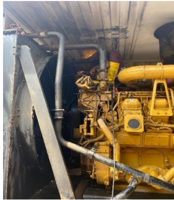
Gambar 4.2 Pembersihan sirip radiator
