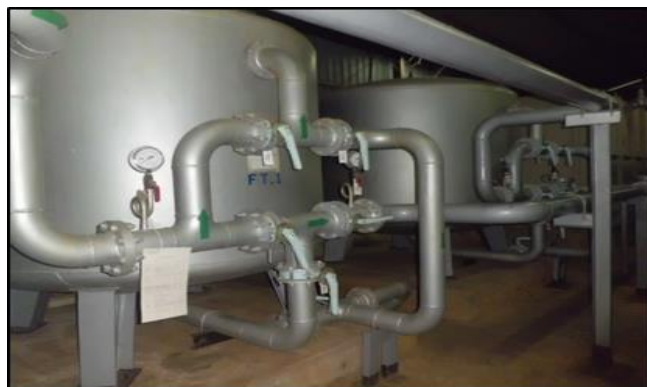
Gambar 3.19 Sand filter tank (Sumber: Unit Layanan PLTA Koto Panjang, 2024)
