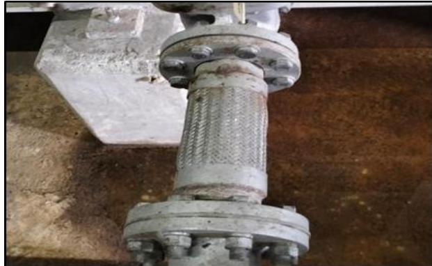
Gambar 3.13 Flexible Joint (Sumber: Unit Layanan PLTA Koto Panjang, 2024)
