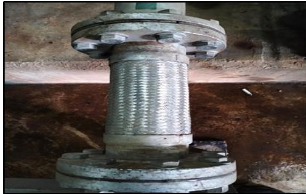
Gambar 3. 18 Flexible joint (Sumber: Unit Layanan PLTA Koto Panjang, 2024)
