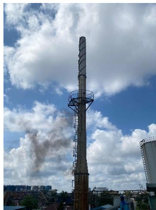
Gambar 3. 8 Cerobong Asap Boiler Advance Sumber : (PT. Kreasijaya Adhikarya)
