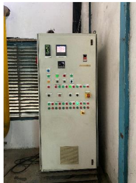
Gambar 3. 4 Panel Control Sumber : (PT. Kreasijaya Adhikarya)
