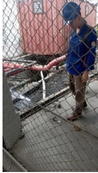
Gambar 2. 14 Drain Water Receiver Tank Sumber : (Dokumentasi, 2024)
