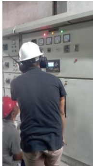
Gambar 2. 44 Commissioning test after service ACB
