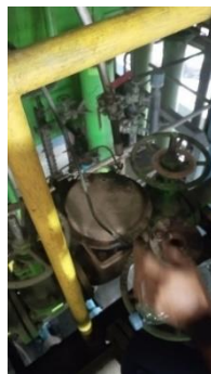
Gambar 2. 26 Proses Mengganti Pneumatic Hose For Air Inlet Control Valve Of Deaerator Turbine Sumber : (Dokumentasi, 2024)
