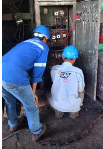
Gambar 2.8 Mengecek Panel Kontrol Sumber: PTPN IV Sei Buatan
