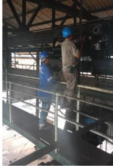
Gambar 2.10 Mengecek Panel Control Hosting Crane Sumber: PTPN IV Sei Buatan
