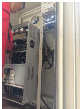
Gambar 2. 40 Repair And Troubleshooting Vsd (Sumber: Dokumentasi Pribadi 2024)
