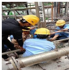
2.17.Ganti Piston Control Valve (Sumber:PT.Indah Kiat Pulp & Paper)
