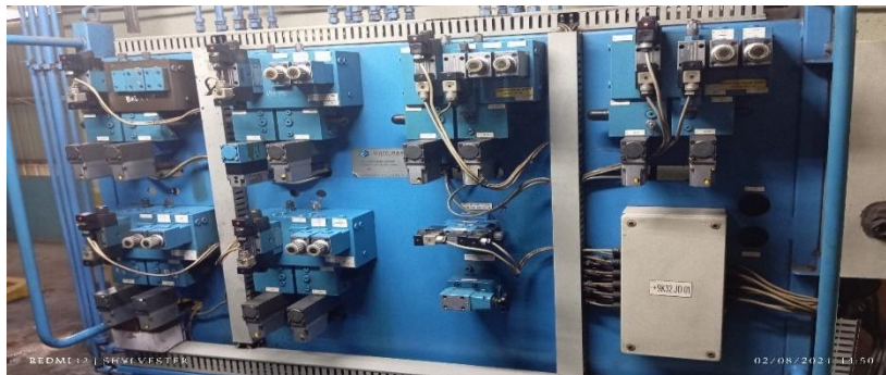
Gambar 2. 14 Gambar Preventive SV hydraulic Section (Sumber : Dokumentasi PT. Indah Kiat Pulp & Paper Perawang 2024.).
