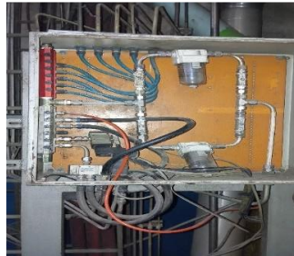
Gambar 2. 3 Gambar Panel control valve
