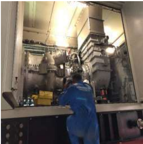
Running Mesin Turbin
