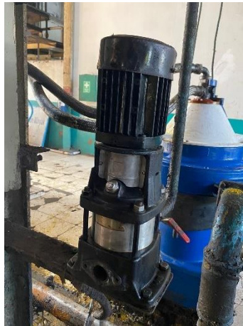
Gambar 3. 6 Water Pump Purifier
