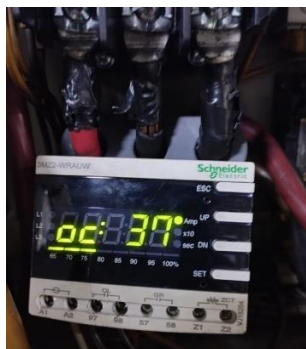
Gambar 3.10 Setting Over Current EOCR (Sumber: Dokumentasi, 2024)
