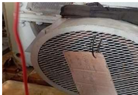
Gambar 2. 55 Check Phase To Phase Generator
