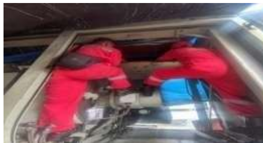
Gambar 2. 19 Connect Kabel Output Generator
