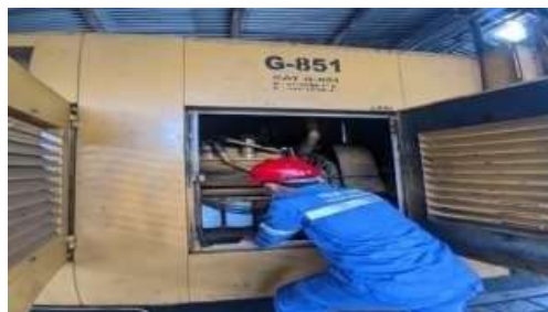
Gambar 2. 6 Prepare Engine Caterpillar
