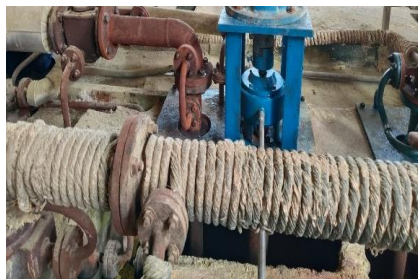
Gambar 4. 12 Pipa Steam (Pemanas) Sumber : PT. UTAKI
