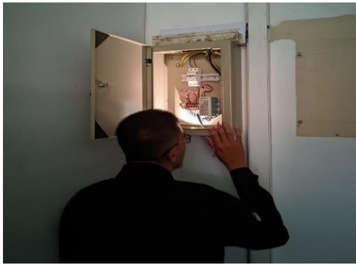
Gambar 3.6 Pengecekan SN (Serial Number) Power Suplay CCTV
