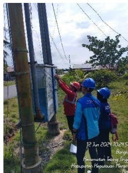
Gambar 2. 9 Memberi tanda Masing – Masing Panel Boks Gardu Distribusi (Sumber: PT. PLN PERSERO ULP Selatpanjang)
