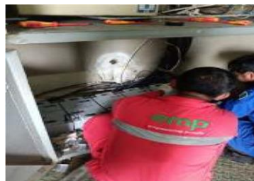
Gambar 2. 31 Check Charger Baterai 12V
