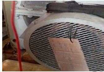
Gambar 2. 55 Check Phase To Phase Generator Sumber: Data Olahan 2024
