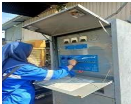
Gambar 2. 30 Disconnect Power Loadbank Sumber: Data Olahan 2024
