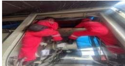
Gambar 2. 19 Connect Kabel Output Generator SumberData Olahan 2024
