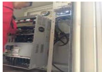
Gambar 2. 40 Repair And Troubleshooting Vsd Sumber: Data Olahan 2024
