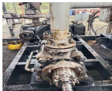
Gambar 4. 17 Main oil pump p-365 (COTP) Sumber.Dokumentasi
