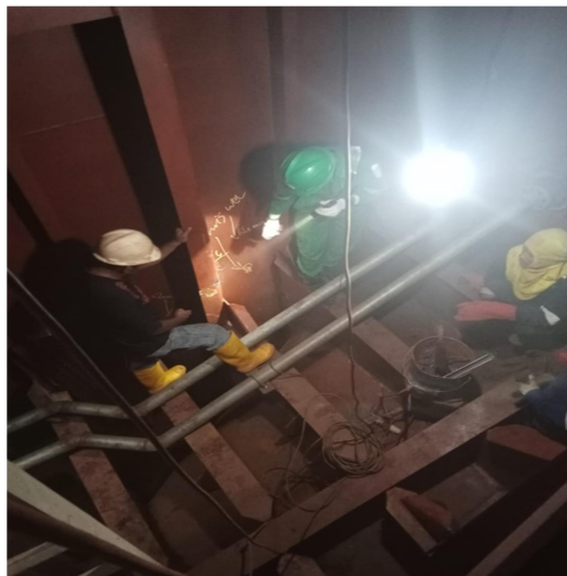
Gambar 2.45 Fresh Water Tank
