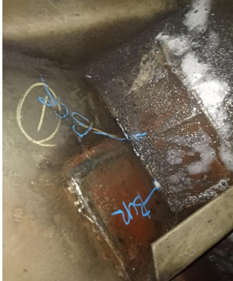
Gambar 2.36 kebocoran Wing tank
