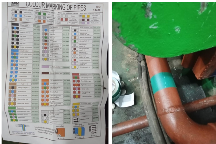
Gambar 2.31 Colour Marking of pipes
