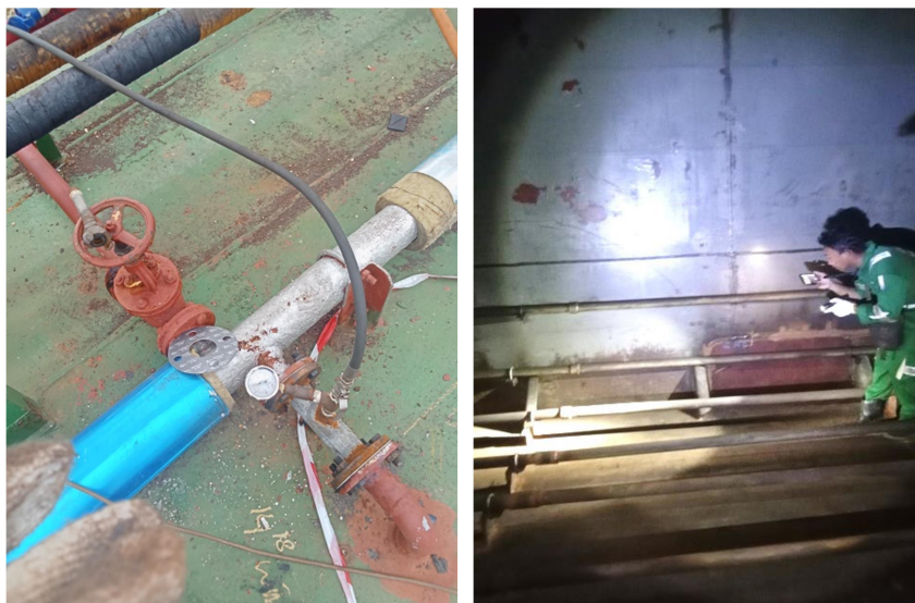
Gambar 2.59 Pipa Steam Boiler
