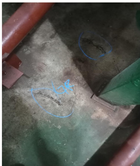
Gambar 2.35 Visual W.I Tank Top Engine Room
