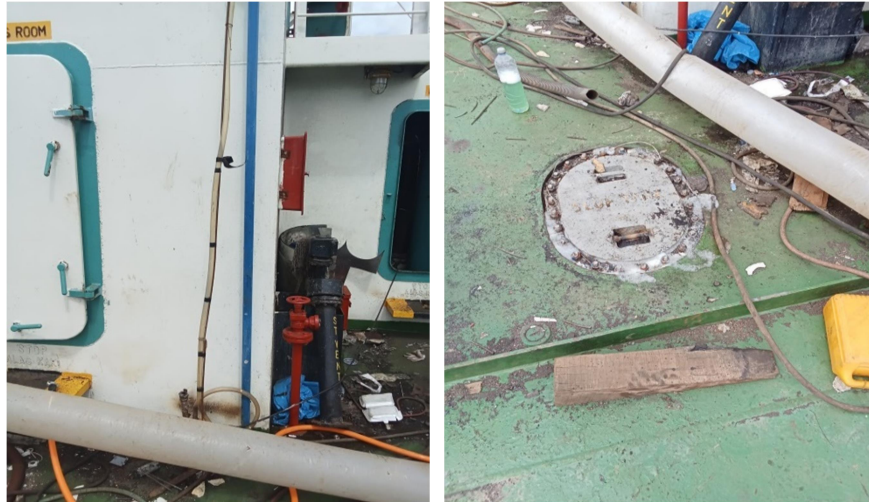
Gambar 2.32 Air Test Slop Tank
