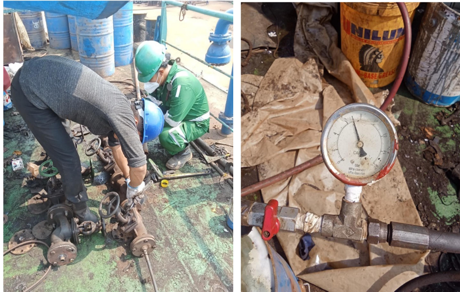
Gambar 2.26 Hydro Test Valve
