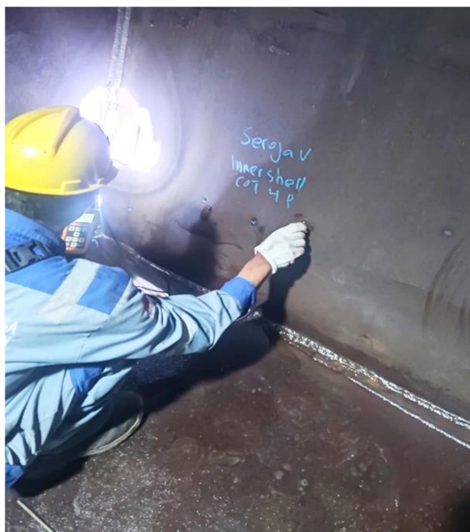
Gambar 2.99 UT Thickness Inner Shell
