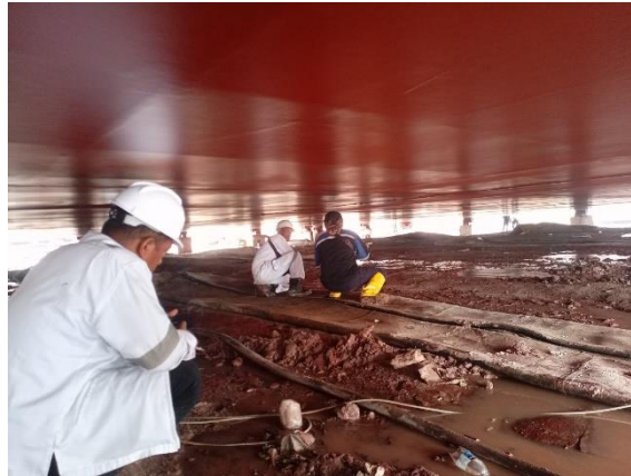
Gambar 2. 42 Visual Inspect Bottom hull 25
