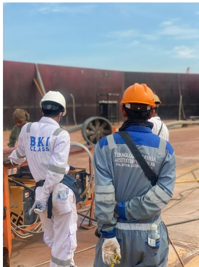
Gambar 2. 35 External air pressure test tank
