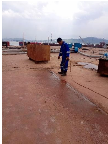
Gambar 2. 13 external air test
