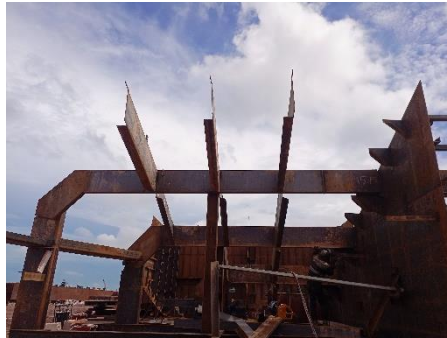
Gambar 2. 86 Misalignment Bottom girder starboard
