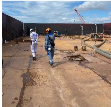
Gambar 2. 34 External air pressure test tank
