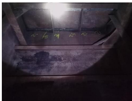
Gambar 3. 23 Markingan di area bocor ( internal air test )
