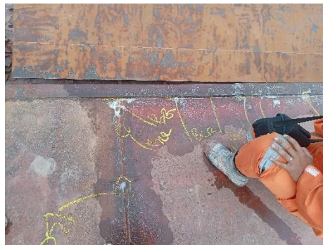
Gambar 3. 25 Markingan di area bocor ( external air test )
